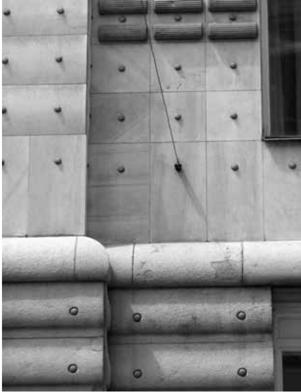
Ill. 5. Facade detail (marble slabs) of the Postsparkasse building (source: photo by author, 2015).
