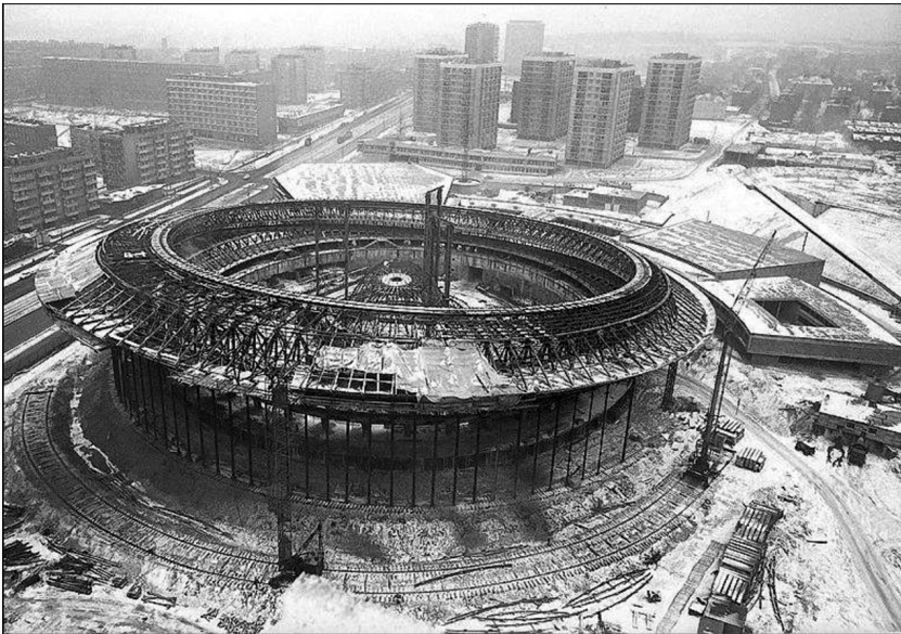
III. 2. Spatial structure of the “Spodek Arena” in Katowice – construction phase of the facility, the archive of “Spodek Arena”.
