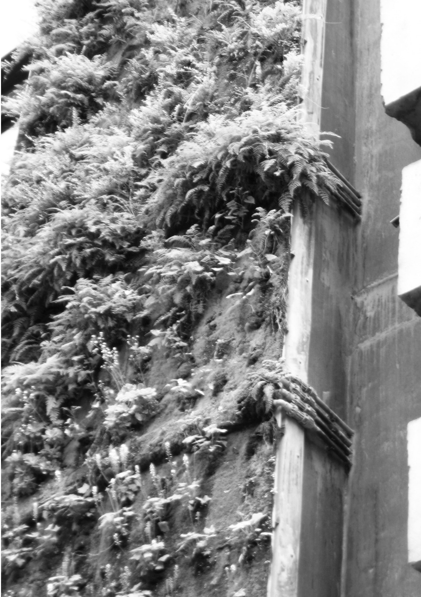
Ill. 3. Musée du Quai Branly (arch. J. Nouvel, 2006), Paris, France. A detail shows the installation necessary for watering plants in the space between the green wall and the neighboring tenement house. The pipes remove the spell of self-sustainable wall greenery, photo by R. Mikielwicz, 2010.
