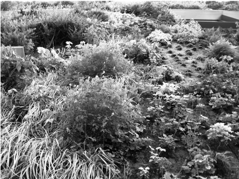
III. 2. Musée du Quai Branly (J. Nouvel, 2006), Paris, France. A detail of the green wall shows problems with the greenery on the wall, photo by R. Mikielewicz, 2010.
