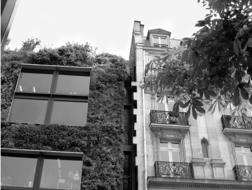
III. 1. Musée du Quai Branly (J. Nouvel, 2006), Paris, France. The design of the link between the most famous green wall, designed by Patric Blanc, and the neighboring 19th-century tenement house is constrained by the necessity of installation, photo by R. Mikielewicz, 2010.
