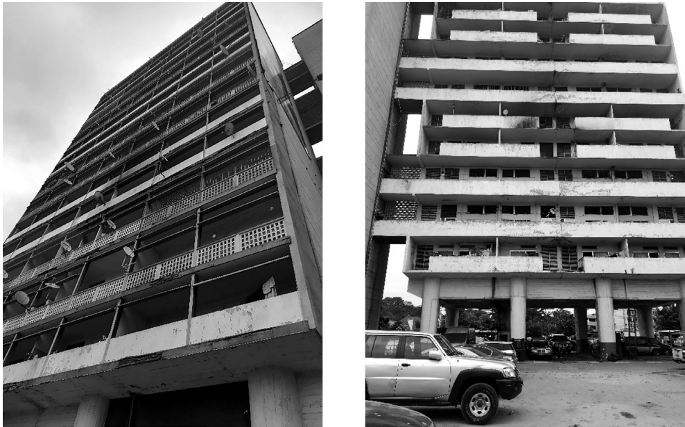
Ill. 2. Detail of the North and South elevations of the Sabena towers, source: Victor Bay, 2022.
