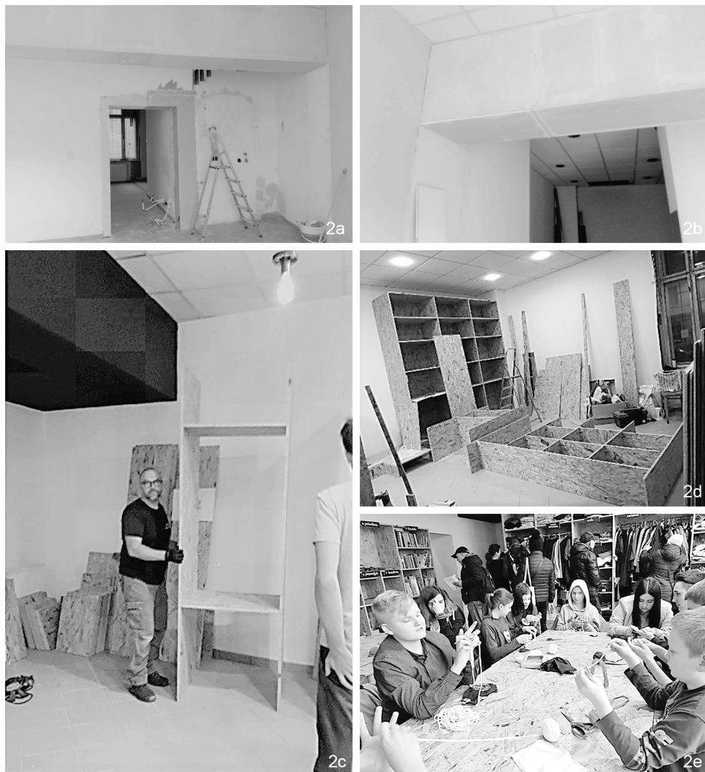
II. 2. Po-Dzielnia , Poznań. Reconstruction and arrangement of the interior of the acquired service premises for the needs of the first free-shop in Poznań; a)–d) author's photo; e) photo Kalina Olejniczak – Po-Dzielnia ; a), b) and d) the design of the reconstruction, interior arrangement and all the furniture was made by students of the Faculty of Architecture at the Poznań University of Technology. A significant part of the finishing materials used during the renovation are recycled materials; c) activities that unite the community around the idea of upcycling: participation of volunteers in construction and finishing works; e) Po-Dzielnia activity: periodic upcycling activities, in the background: cabinets for exchanging clothes, books, house accessories
