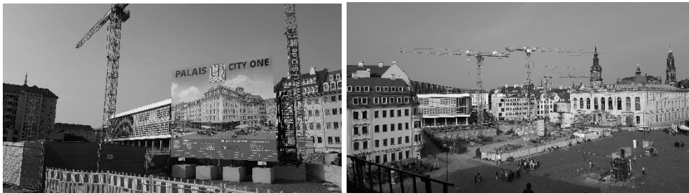
Ill 8. Construction work on the reconstruction of town blocks within Neumarkt, photos by M. Krupa, 2019.
