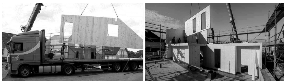
III. 2. Delivery and assembly of CLT elements on the construction site using a crane, source: What is cross laminated timber (CLT)? [in:] Eugen Decker, https://www.eugen-decker.de/en/cross-laminated-timber.html (access: 14.07.2025)
